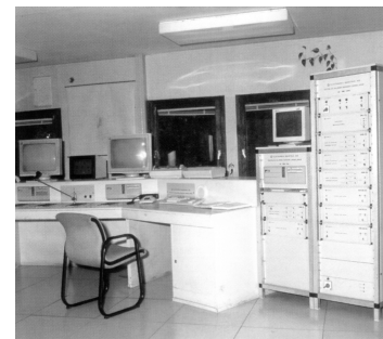
Figure 1. The control centre in rembas mine complex.
